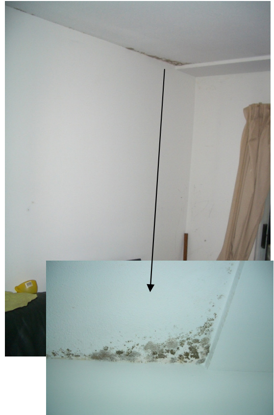
Photograph showing condensation and organic growth on the ceiling of a concrete slab adjacent to an exposed slab edge thermal bridge. Condensation has formed here frequently as a result of colder interior surface temperatures.
